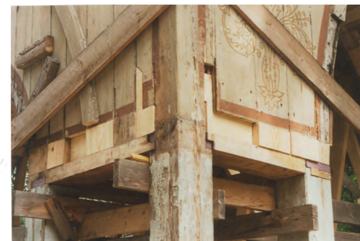
2002, 2nd group of pillars. Prostheses of the facade boards are done on site without dismantling the boards
